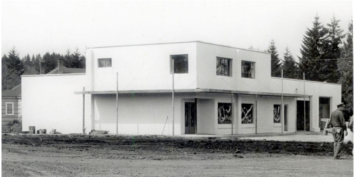
Fred & Evie's new store on South side of Highway 30 as shown during construction in 1951.
